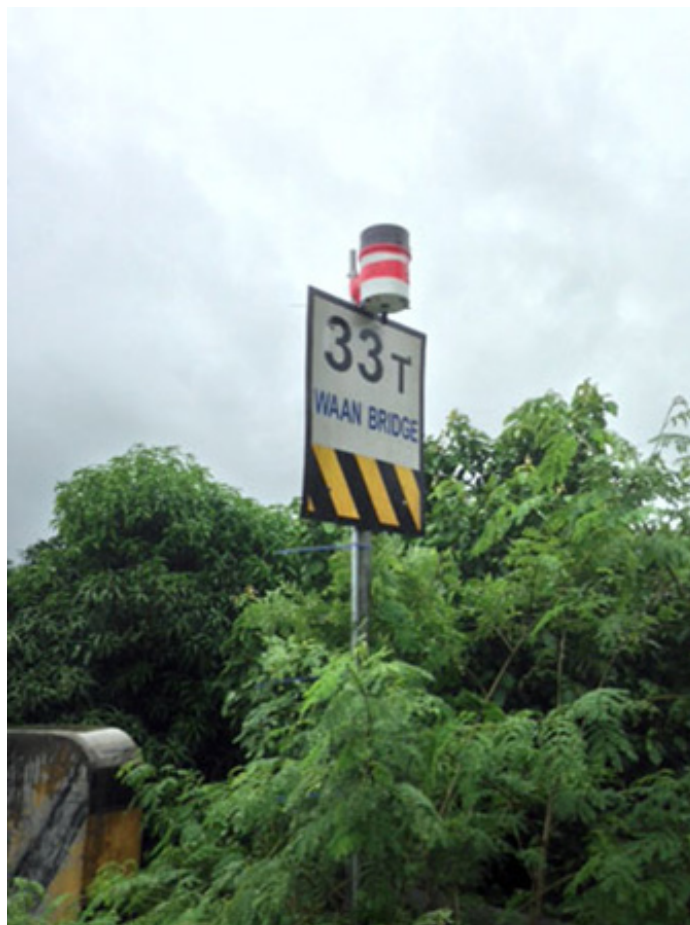
Figure 23. Rain gauge deployment at Waan Bridge, Brgy. Waan, Davao City
