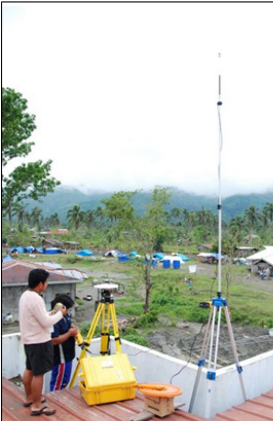
Figure 16. RTK base set up at UP-NB 1 at the roof top of New Bataan Town Hall in Brgy. Fatima, New Bataan, Compostela Valley.
