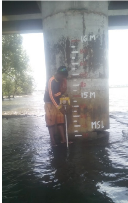
Figure 40. Water-level markings on Can-Avid Bridge
