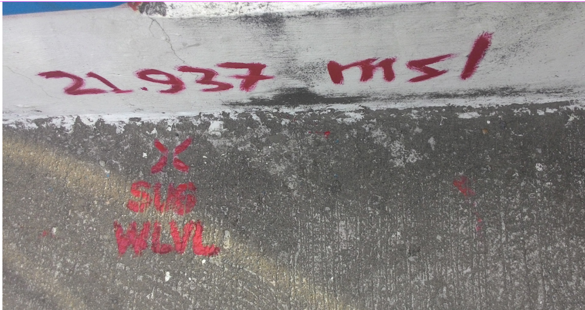
Figure 40. Water level markings on the Subangdaku Bridge 2 railings
