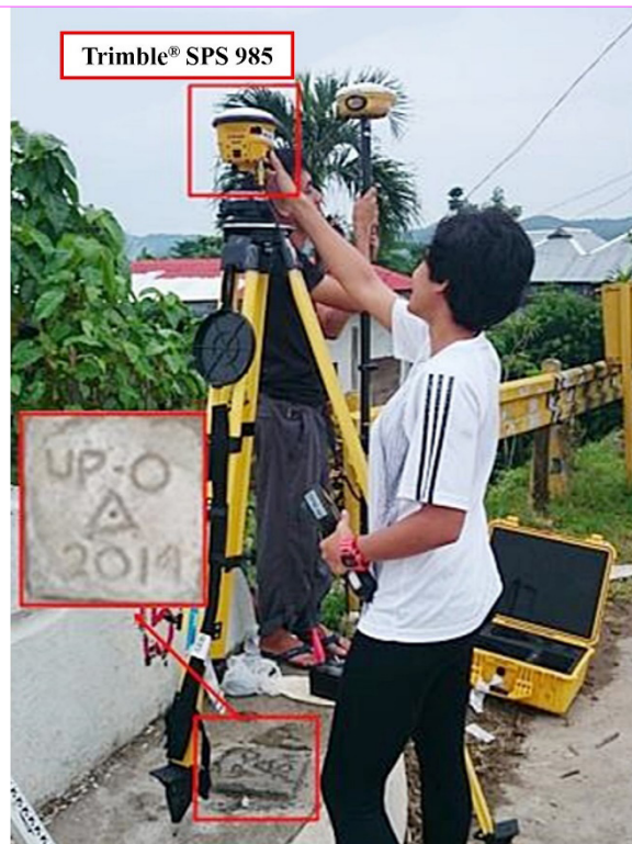
Figure 38. GNSS receiver set-up, Trimble® SPS 985, at UP-O, an established control point, located at the bridge approach of the Ormoc Merida Bridge along the Ormoc-Merida-Isabel-Palompon Road in Barangay. Liloan, Ormoc City, Leyte
