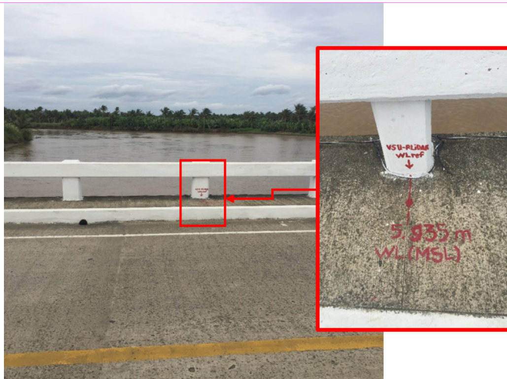
Figure 41. Water-level markings on Pambujan Bridge.
