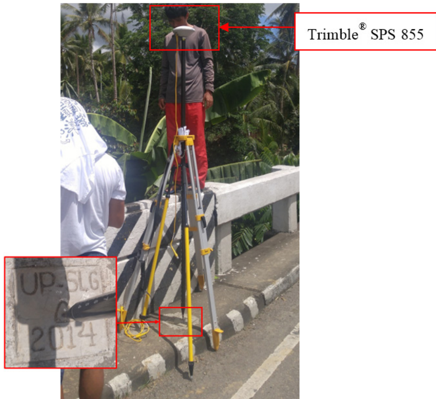
Figure 30. GNSS base set up, Trimble® SPS 855, at UP-SLG, located at the approach of the left side of Silaga Bridge in Brgy. Tominamos, Municipality of Santa Rita, Samar
