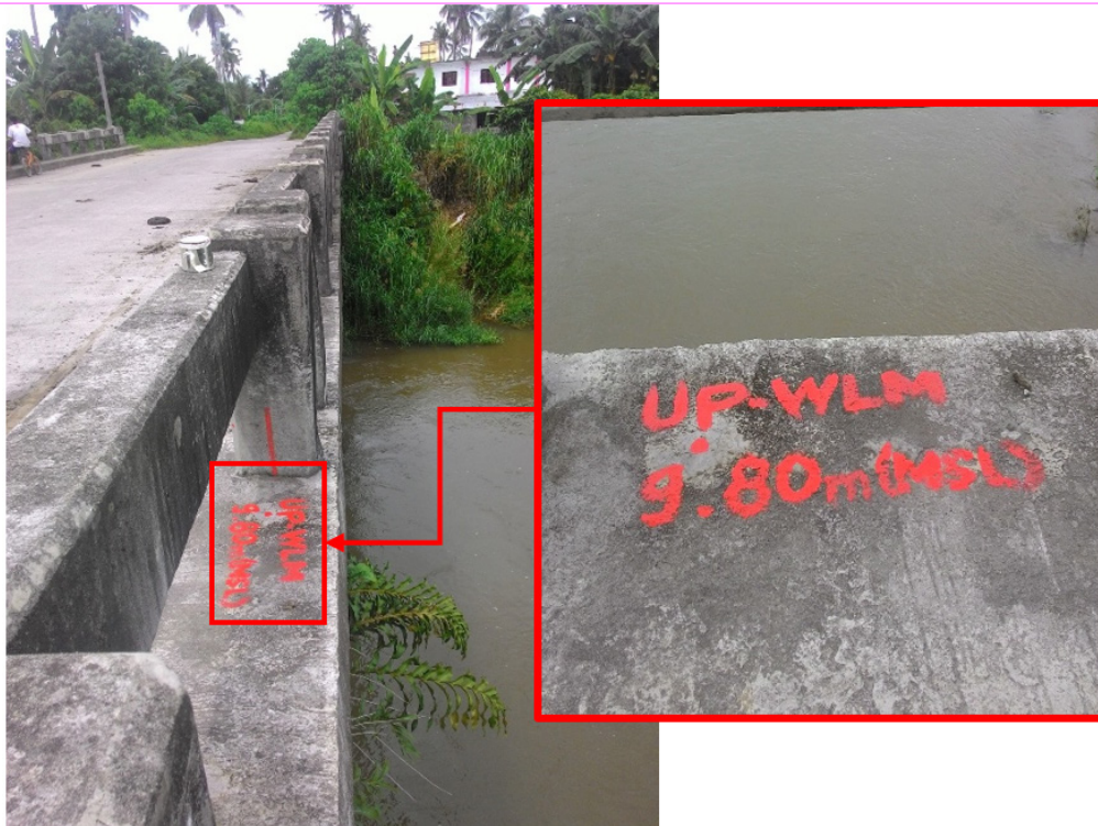
Figure 50. Water-level markings on Sta. Elena Bridge
