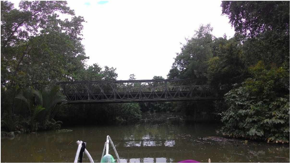
Figure 46. Water-level markings on Tugas Bridge
