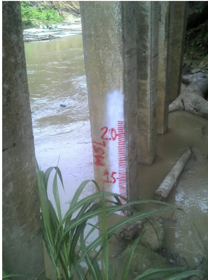
Figure 41. Water level markings on the post of the Dolor Bridge
