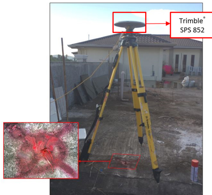
Figure 31. GNSS base receiver set-up, Trimble® SPS 852 at RB-1, located at the roof top of Asia Blooms Hotel, Brgy. Patimbao, Sta. Cruz, Laguna
