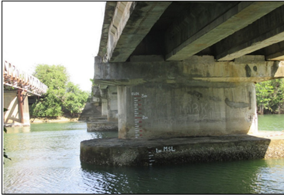
Figure 41. Water-level markings on Iwahig Penal Bridge
