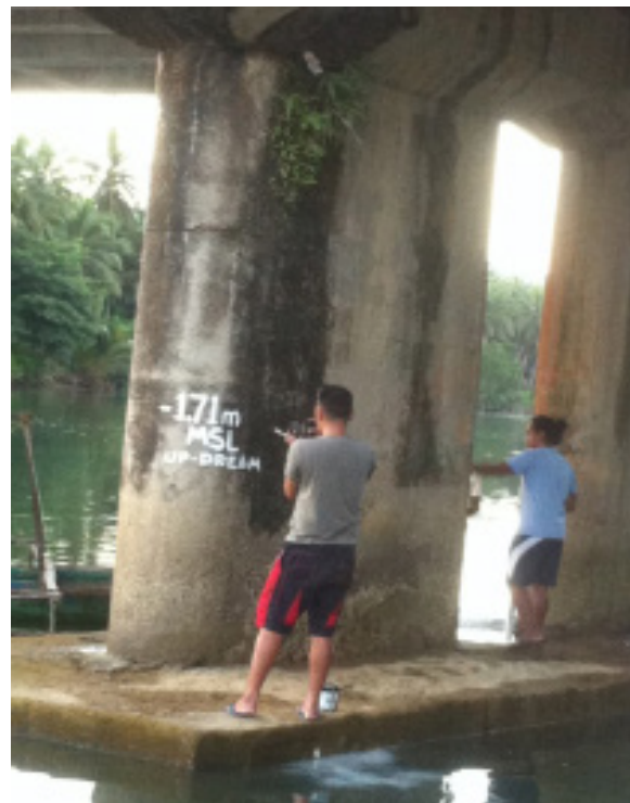
Figure 39. Water-level markings on the post of Babuyan Bridge
