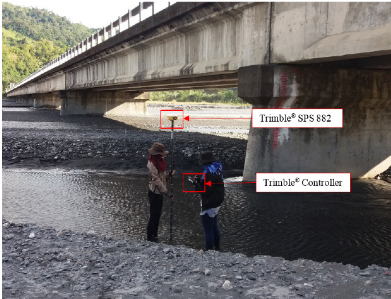
Figure 40. Bridge cross-section acquisition along the upstream side of Amnay Bridge, Brgy. Pagasa, Municipality of Sablayan
