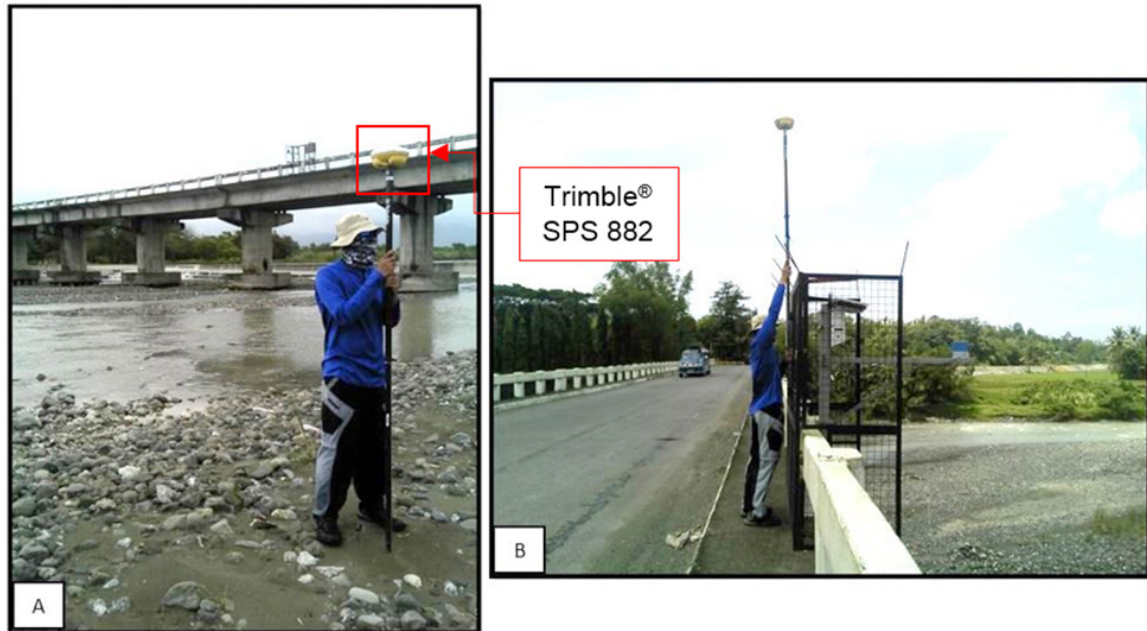
Figure 41. (A)Cross section survey and (B)As-built survey in Tipuluan Bridge, Municipality of Sibalom2.
