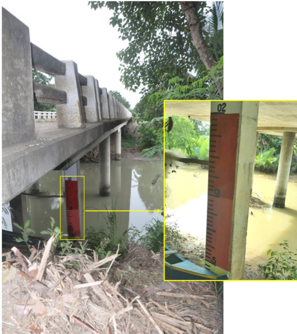
Figure 39. Existing water level mark at one of the piers of Danao Bridge
