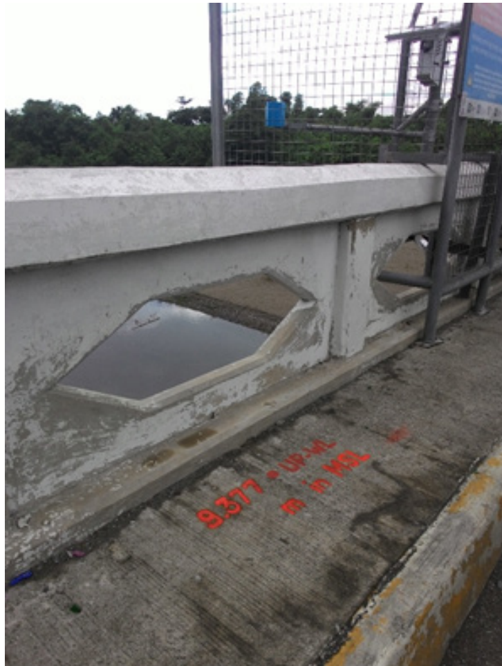
Figure 40. Water-level markings on the deck of Santa Cruz Bridge
