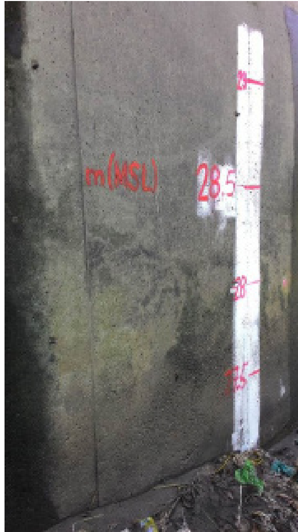
Figure 41. Water level markings on the side of the pier in Daang Hari Bridge
