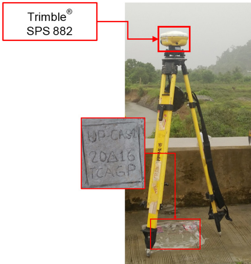
Figure 36. GNSS receiver setup, Trimble® SPS 882, at UP-CAS-2, located at the approach of Casalugan Bridge in Brgy. Culat, Municipality of Casiguran, Aurora
