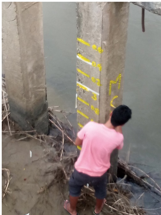
Figure 48. Water-level markings on Casalugan Bridge
