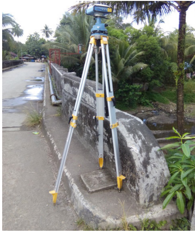
Figure 31. GNSS receiver set up, South® S86T, at SRN-102, located at the approach of Bridge in Brgy. Poblacion, Sison, Province of Surigao del Norte.
