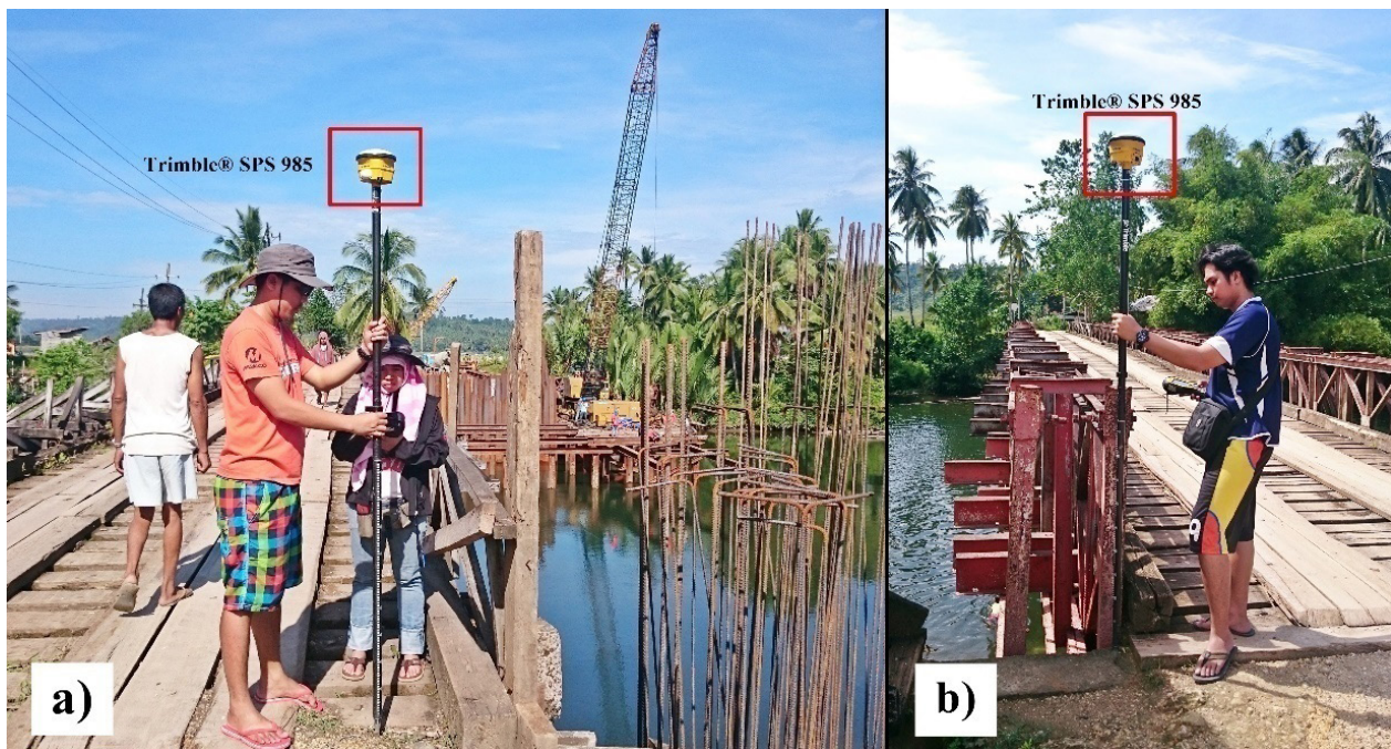
Figure 44. As-built at (a) Bagnan Bridge (b) and Burboanan Bridge in Bislig City, Surigao del Sur
