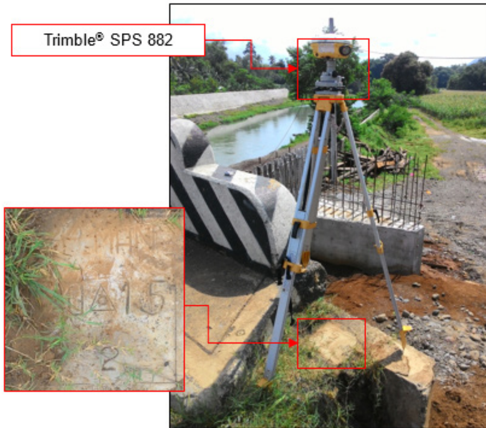
Figure 37. GNSS receiver set up, Trimble® SPS 882, at UP_MAN -2, located near the approach of Manupali Bridge in Brgy. Bangcud, Malaybalay City, Province of Bukidnon
