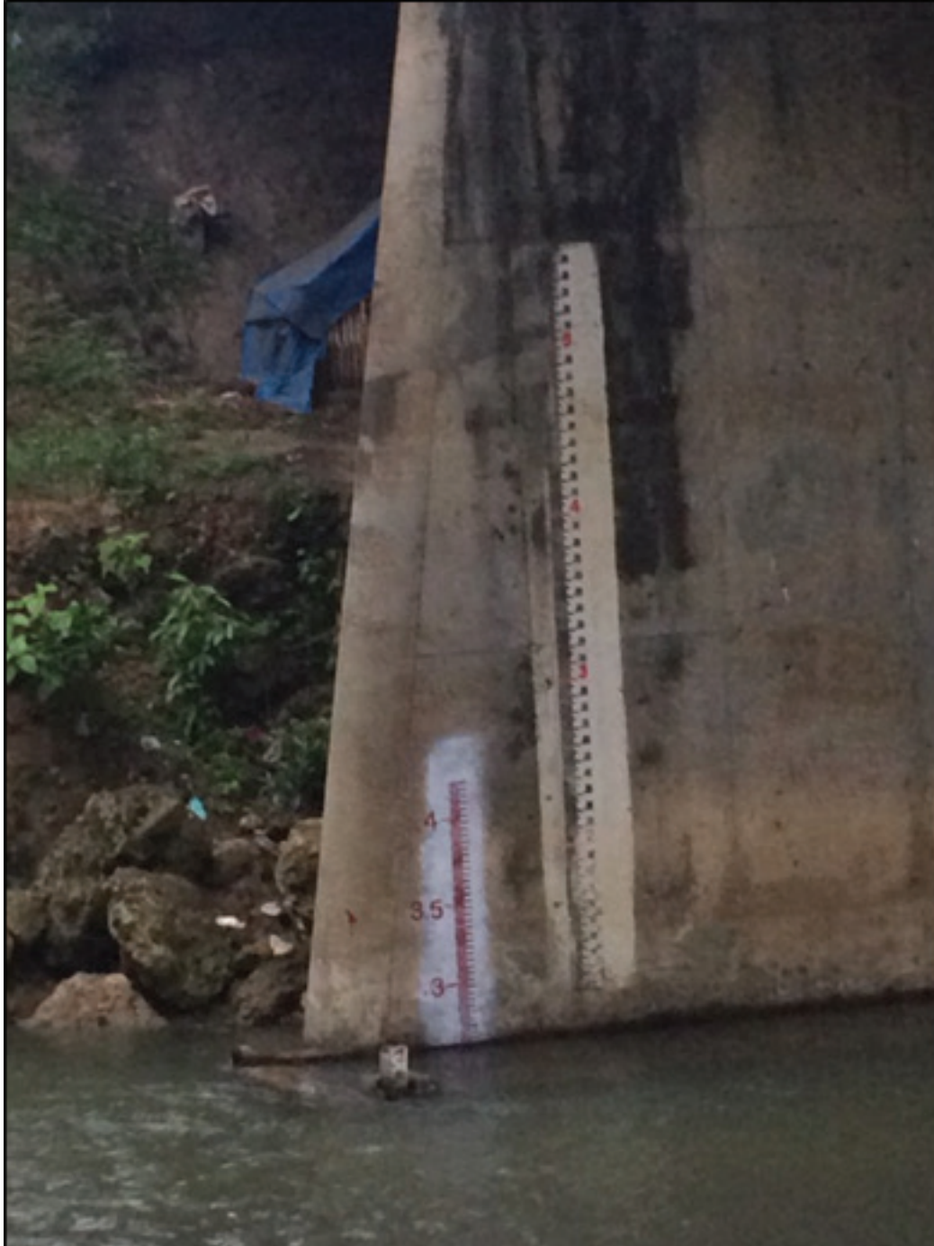
Figure 38. Water level mark at the pier of Alubijid Bridge.
