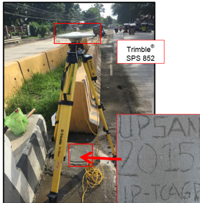
Figure 34. GNSS base set up, Trimble® SPS 882, at UP-SAN, located at the approach of Sanito Bridge in Brgy. Sanito, Municipality of Ipil, Zamboanga Sibugay
