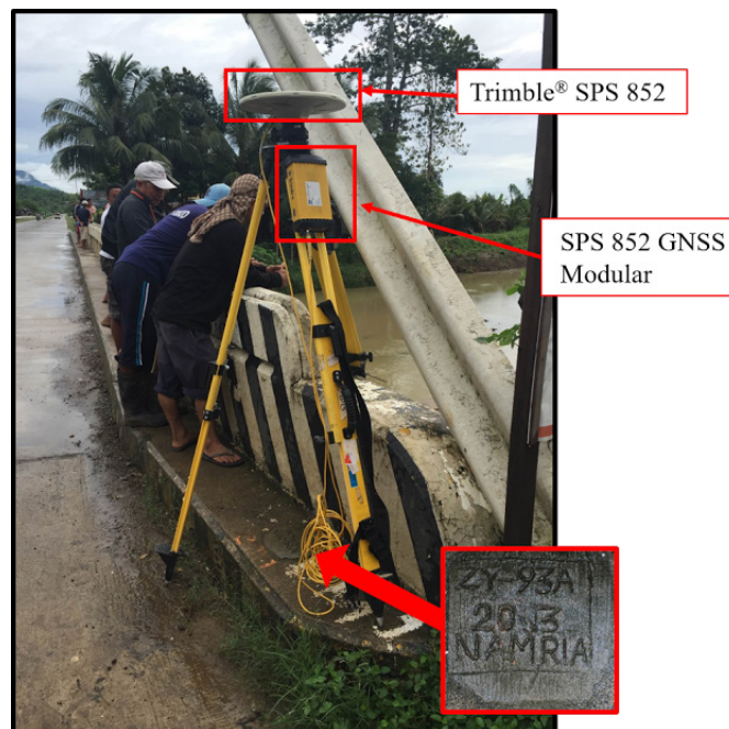
Figure 36. GNSS base set up, Trimble® SPS 852, at ZY-93A, located at the approach of Tupilac Bridge, in Brgy. Tupilac, Municipality of Roseller Lim, Zamboanga Sibugay
