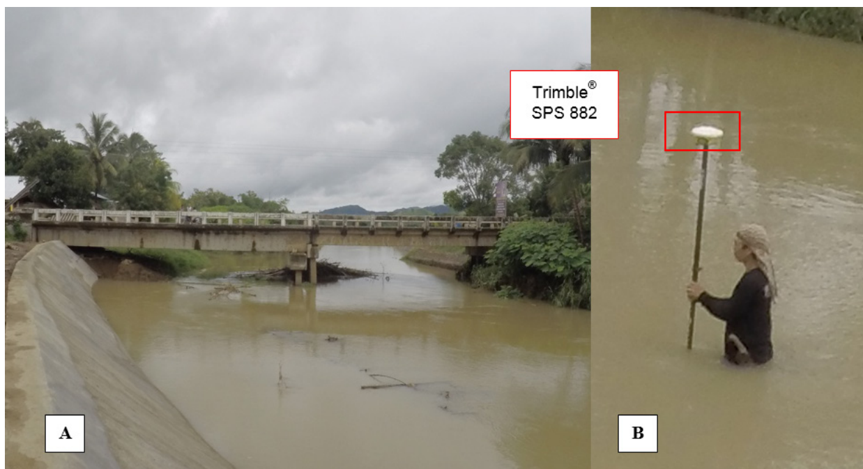
Figure 39. A) Tupilac Bridge facing upstream, and B) Bridge cross-section survey of Tupilac Bridge
