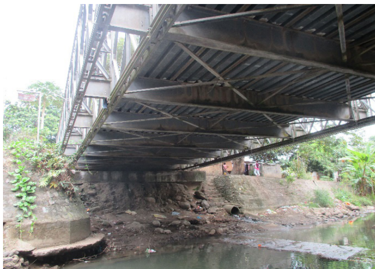
Figure 2. Sewer pipes draining into the river
