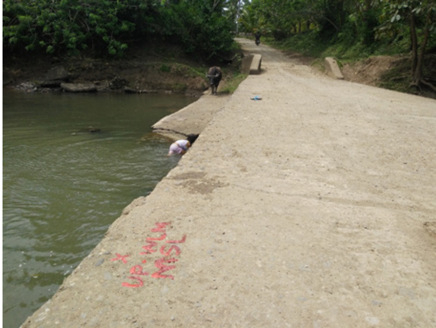
Figure 46. Water-level markings on Malbag Culvert
