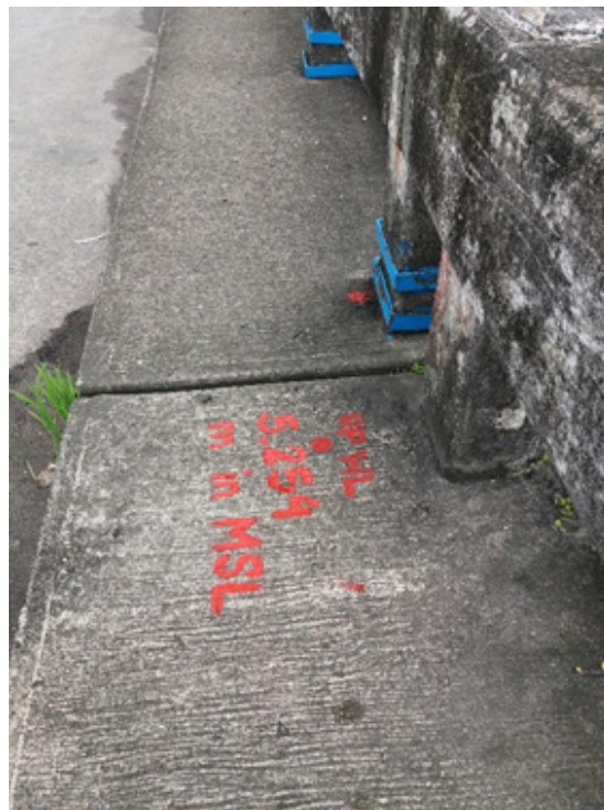
Figure 41. Water-level markings on Mocong Bridge
